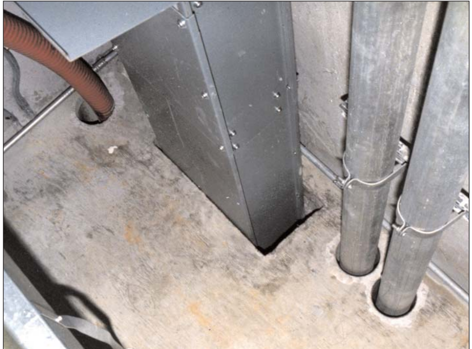
Cable penetrations in parking garages were air sealed
