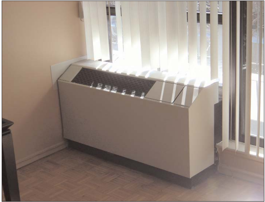
Horizontal air source heat pump in one-bedroom suite
